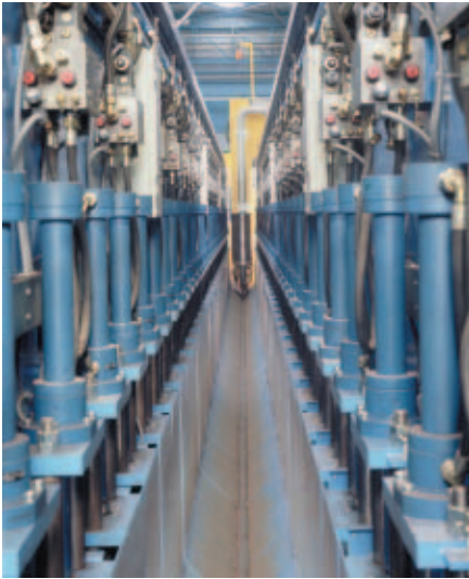
View into milling-drain of milling-portal; right and left hydraulic plate clamping devices; laser-hybrid welding head in background
